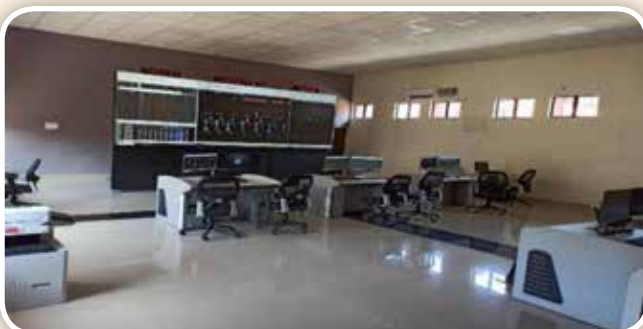
Energy Management Centre has been established by PGCIL
