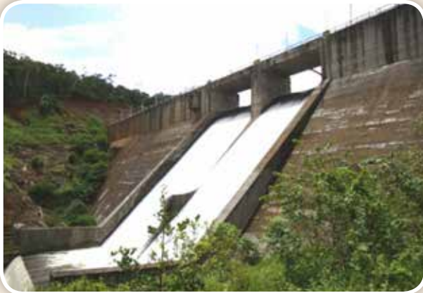
5.25 MW Small Hydro plant functioning at Diglipur, North Andaman generates around 12 MU annually.
