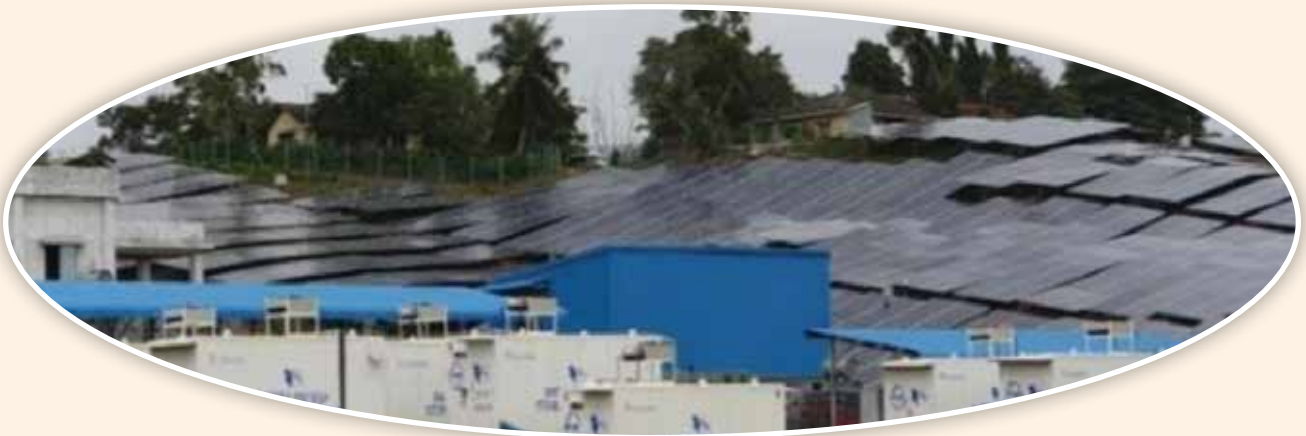
20 MW ground mounted solar plant Functioning at Atampahad/Dollygunj since July 2020 which generates around 12-13 MU annually.
