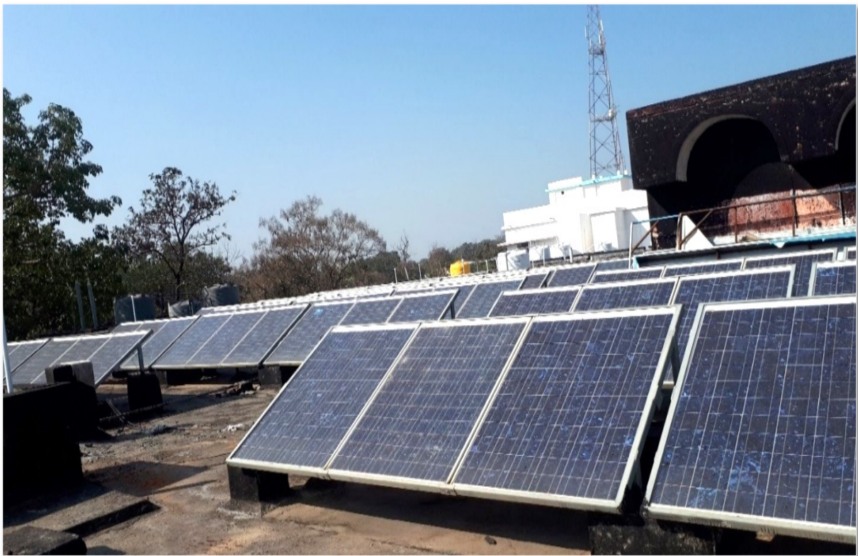
Figure 2: Solar Panel, District Healthcare Facility, Bijapur, Chhattisgarh
