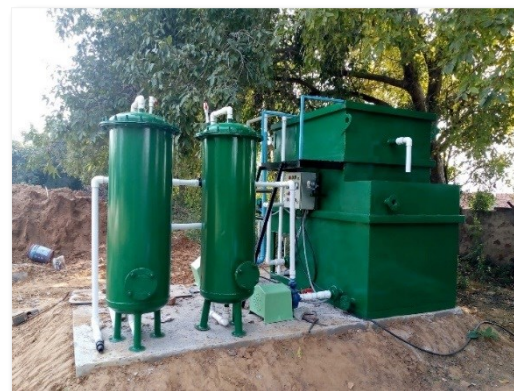
Figure 22: Sewage Treatment Plant
