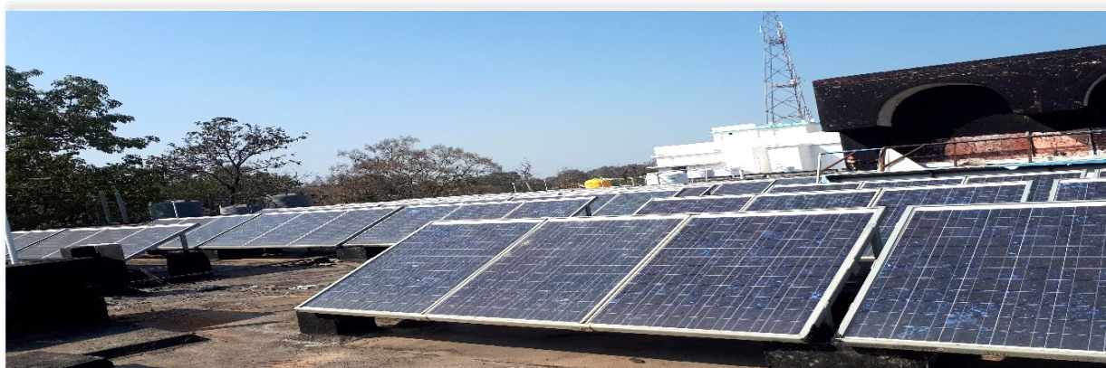
Figure 5: Solar Panel, District Healthcare Facility, Bijapur, Chhattisgarh
