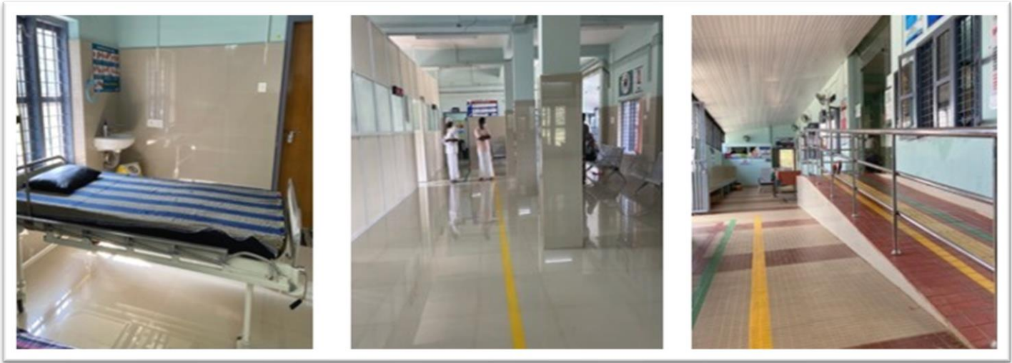
Tiled floors and elevated ramps to reduce impact of flood waters and ensure continued health care delivery, features of a flood-resilient health facility
